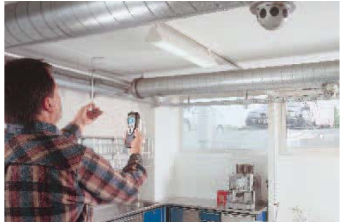
Measuring outlet air
